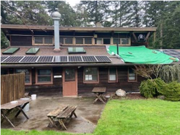
Roof damage and area to be replaced
